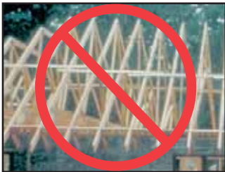
Above: Improper bracing scheme - Continuous TCTLR with no Diagonal Bracing - WHAT NOT TO DO PHOTO B2-6
